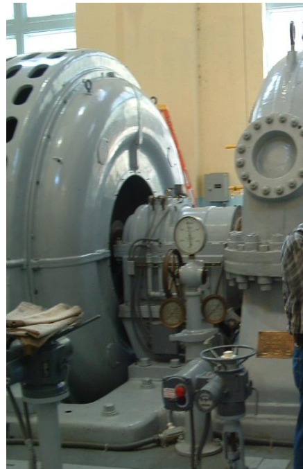
LaGrande 6MW Turbine Generator
