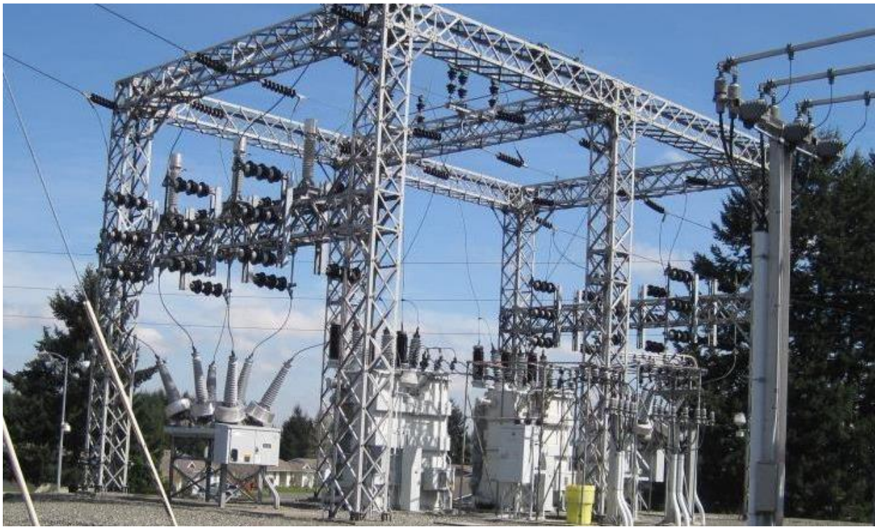
Figure 6-28 Electrical Substation in Tacoma (courtesy of Tacoma Power)
